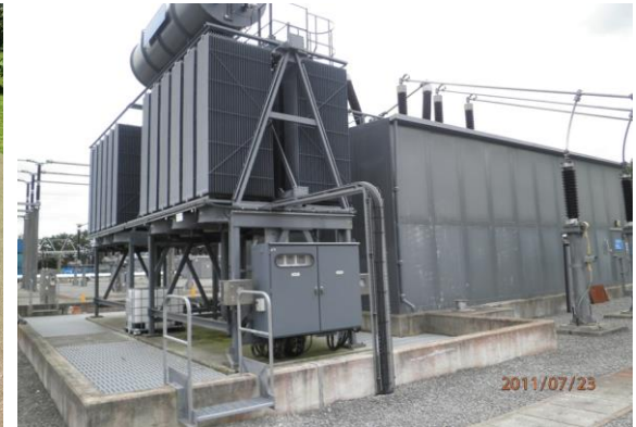
400 kV Power Transformer
